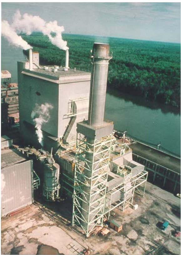
Figure 10. Black Liquor Recovery Boiler (BRLB)
